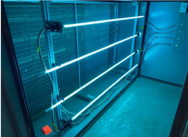
UVC 254nm lighting in air handling unit at 1828 L Street NW, Washington, D.C.
